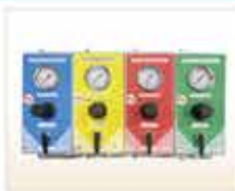
Gas Distribution Panel
